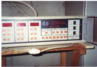
Figure 1. Control unit of drying
